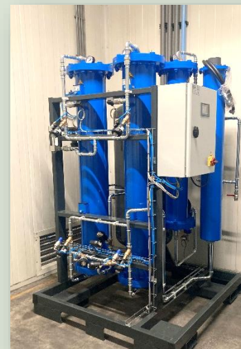
N2 injection system
