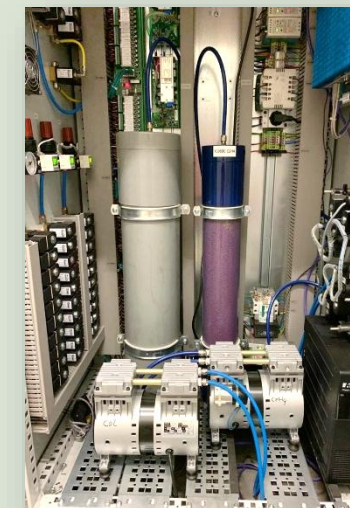
CO2 & Ethylene adsorber
